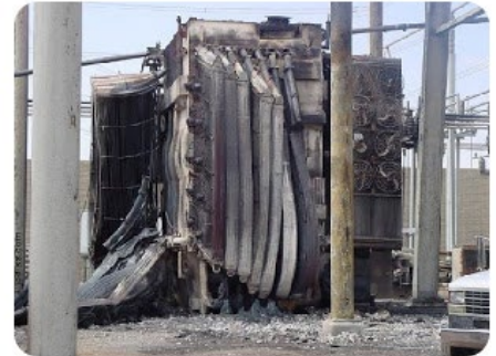
Catastrophic transformer failure
